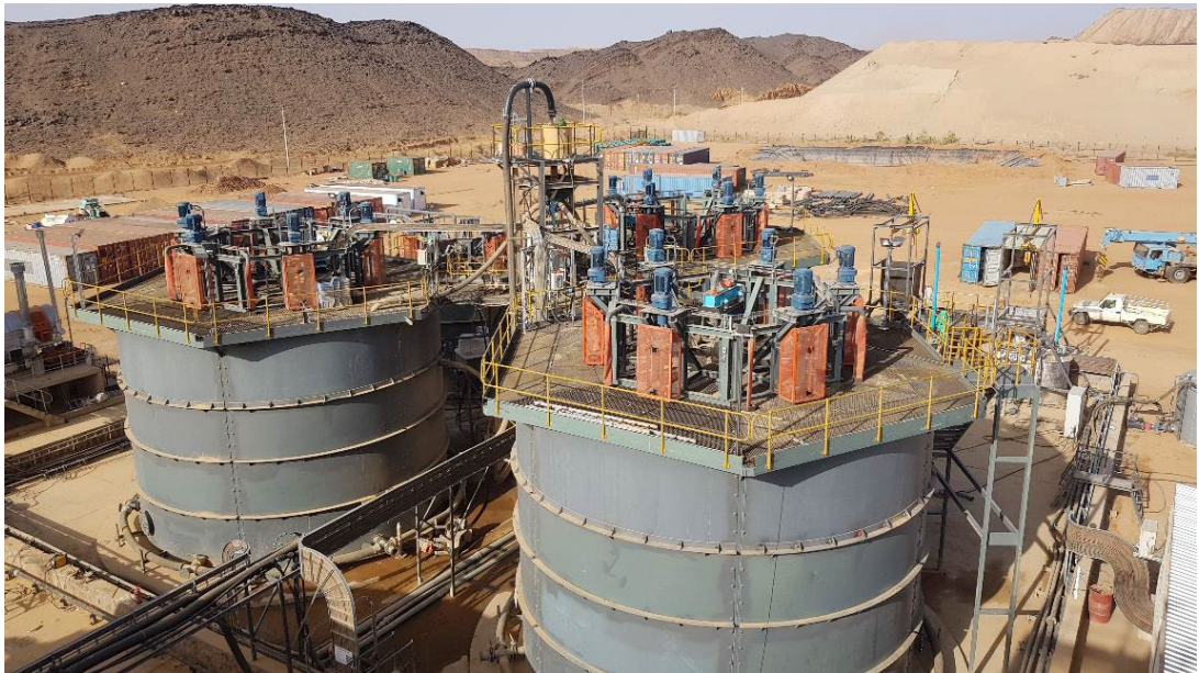
Operational TriTanks prefabricated and installed by APT in North Africa. 395
